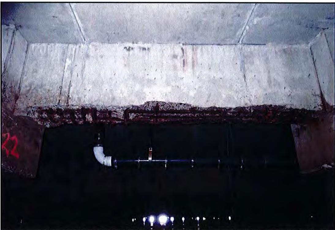
Photo B-28: Concrete beam in the Pier Shed with a full length spall and exposed reinforcement. View looking west at Bent D-bar between Pile Row 8.5 and 8-bar.
