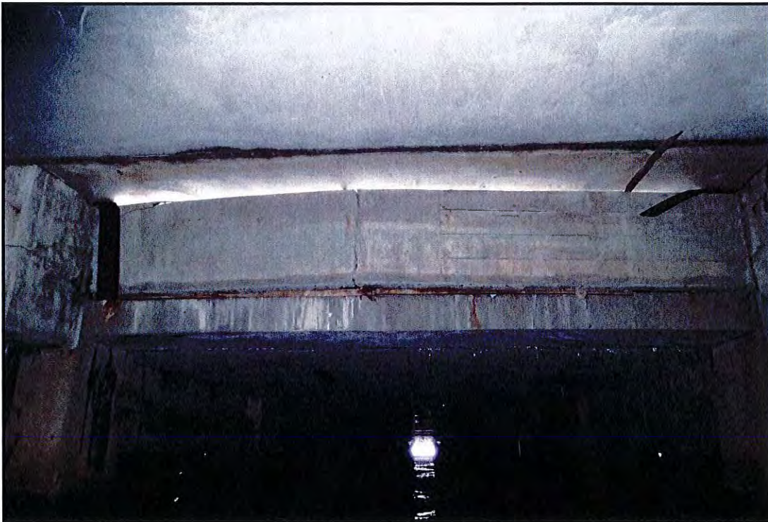
Photo B-29: Concrete closure wall with large vertical crack and deflection View looking north at Pile Row 7-bar between Bent I and I-bar.
