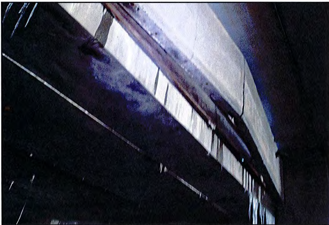
Photo B-30: Concrete closure wall with large vertical crack and deflection View looking east at Pile Row 7-bar between Bent I and I-bar.
