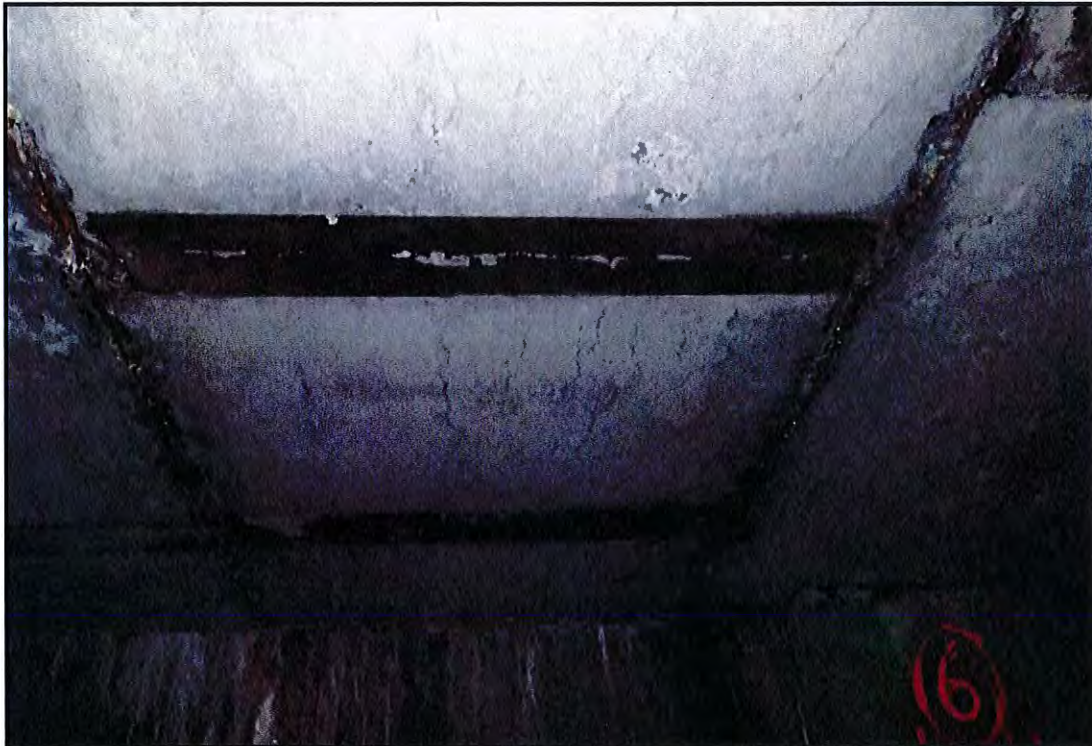
Photo B-33: Typical condition of Court Yard deck soffit with light shrinkage cracks. View looking west between Bent I and I-bar at Pile Row 9-bar.
