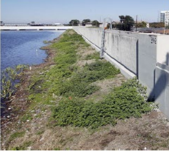
Floodwalls: Permanent or deployable walls used at the shoreline or upland to prevent flooding.
