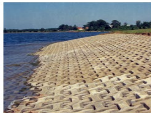
Revetments: Shoreline structures typically made of stone rubble or concrete blocks placed on a sloped surface to protect the underlying soil from erosion and reduce the force of wave action.
