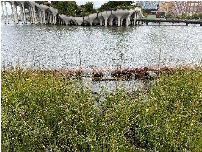
Fig. 5 | One of two inlets where reef balls were deployed at the Gansevoort salt marsh, tied to bolts driven into the rock.
